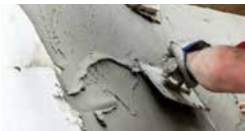
DryMix Building Materials Processing
